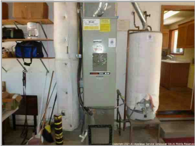
Furnace (gas)/Hot Water (gas) (Location: Two-Car Garage)
