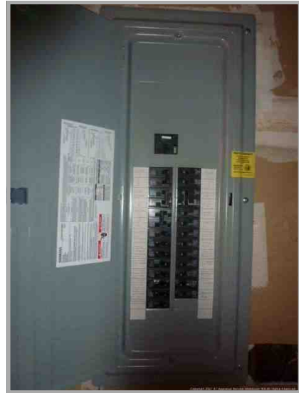
Circuit Breaker Panel; garage
